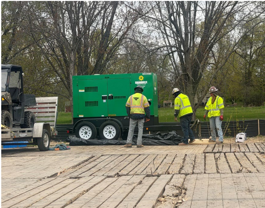
Facing north near MP 3.42, InterCon placed the generator in secondary containment
