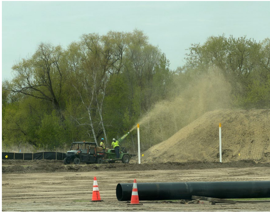
Facing southwest near MP3.5, InterCon stabilizing the topsoil pile with certified weed-free straw
