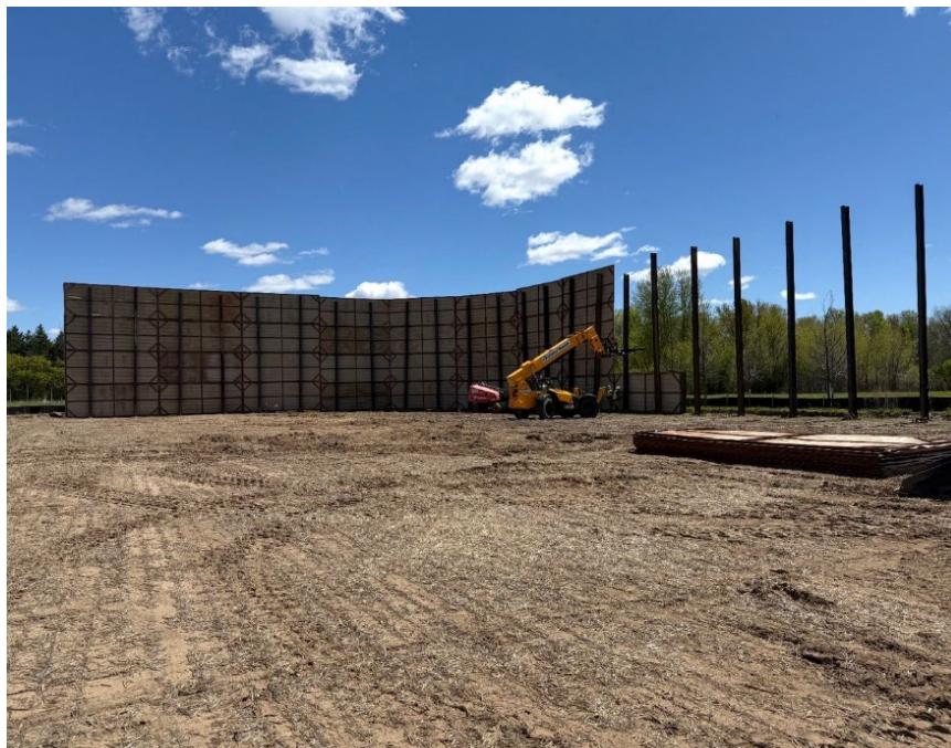
Facing east near MP 3.0, InterCon installing the sound wall on HDD P4-5 exit side
