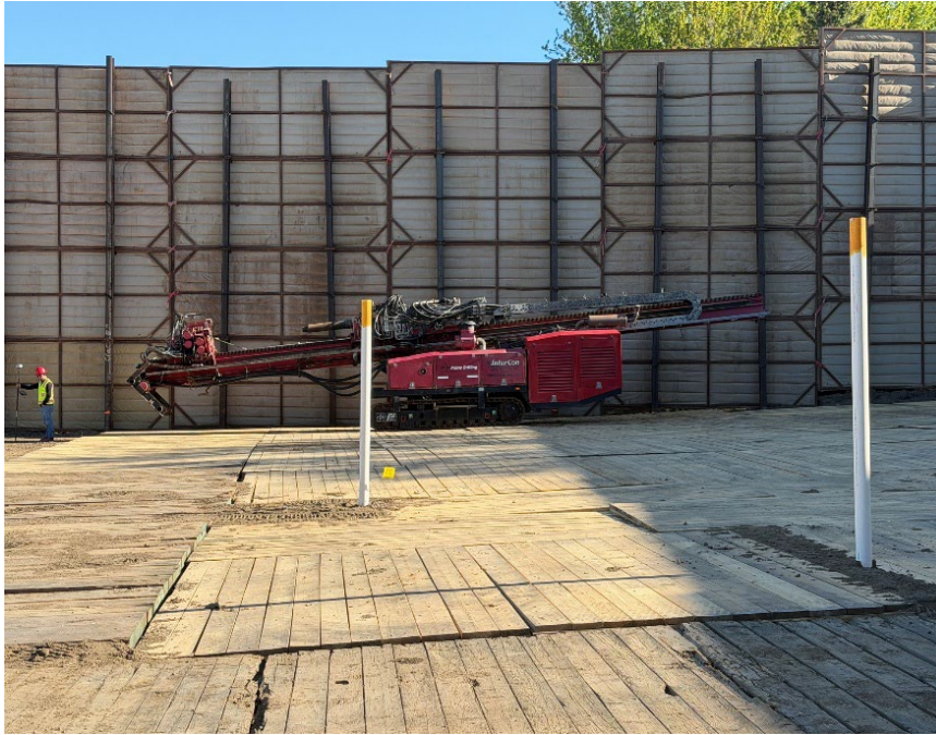
Facing north near MP 2.4, drill rig delivered to HDD P4-5 entry side
