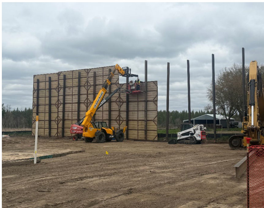
Facing north near MP 2.4, InterCon installing the soundwalls at entry side of HDD P4-5
